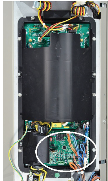
Figure 34 – Panneau de commande AOC (Application Operational Control)
