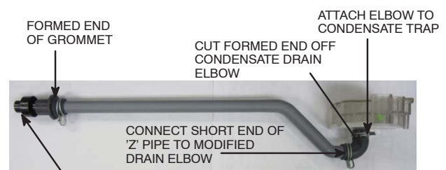
FACTORY SUPPLIED 1/2-IN. CPVC TO 3/4-IN. PVC ADAPTER TOP VIEW DRAIN ELBOW "Z" DISCHARGE PIPE FOR LEFT SIDE DRAIN IS ROUTED BEHIND INDUCER
