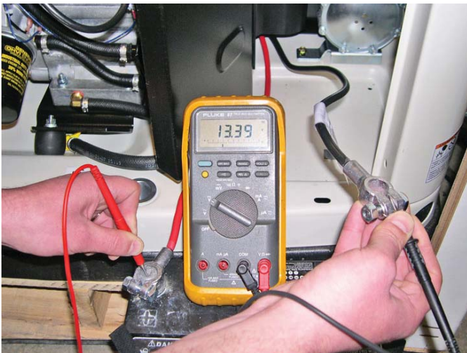
Figure 3.12 — Measurement of Charger Output with Battery Disconnected
