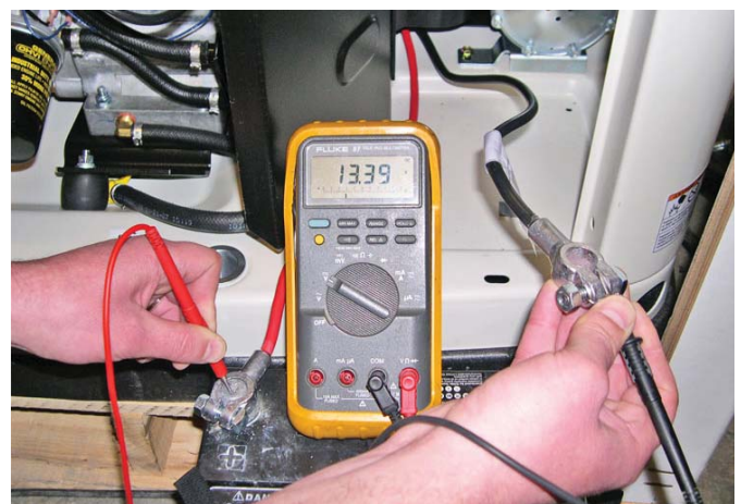
Figure 2.3 — Measurement of Charger Output with Battery Disconnected
