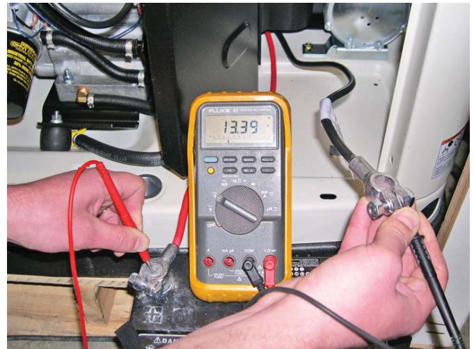
Figure 4.8 — Measurement of Charger Output with Battery Disconnected
