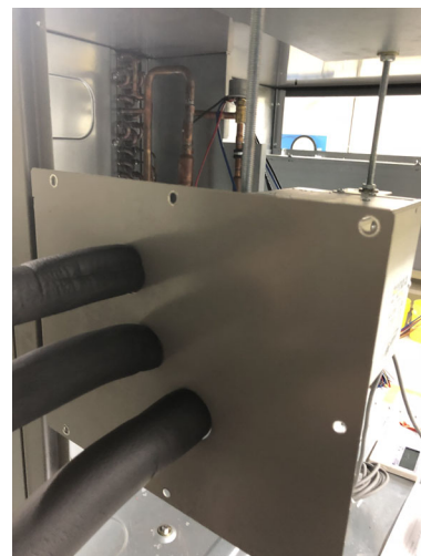
Fig. 51 - Knockouts and Line Sets
