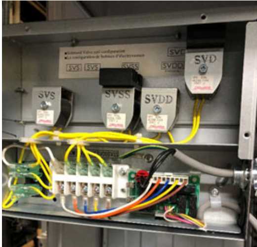
Fig. 52 - FS Box with Panel Removed
